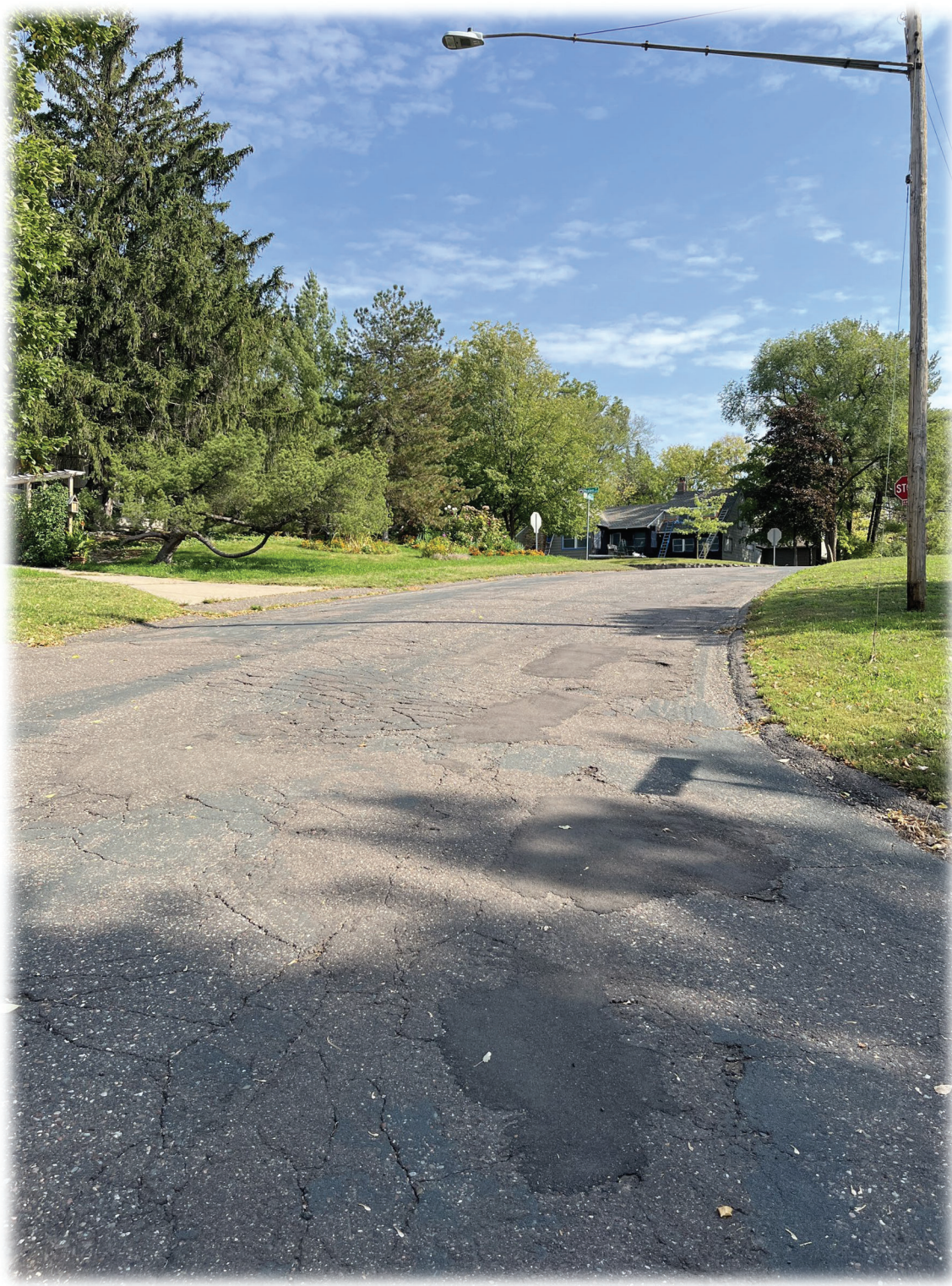
FIGURE 5: Pavement Condition of the East Shore Drive Area Streets
