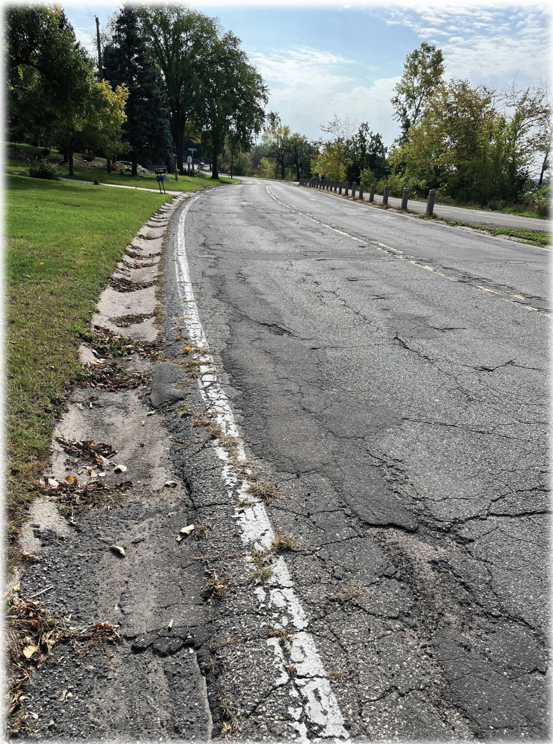
FIGURE 3: Pavement Condition of the East Shore Drive Area Streets
