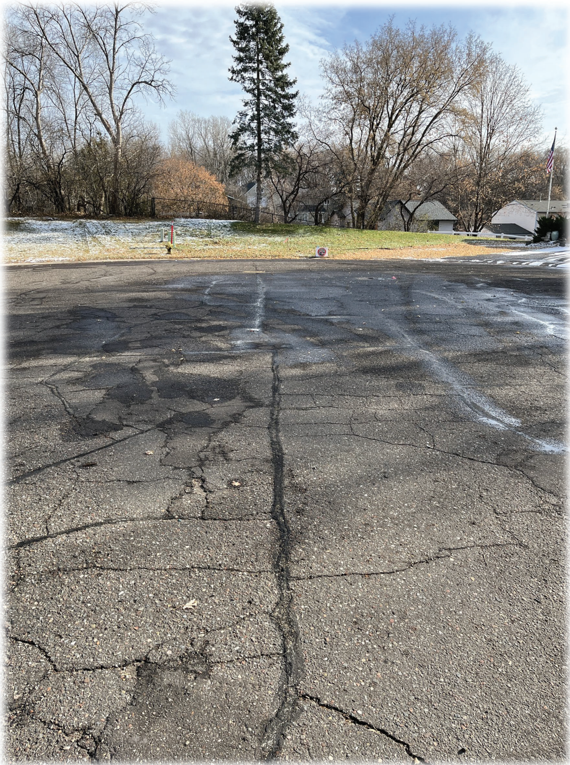
FIGURE 8: Pavement Condition of the Cypress-Maplewood Drive Area Streets
