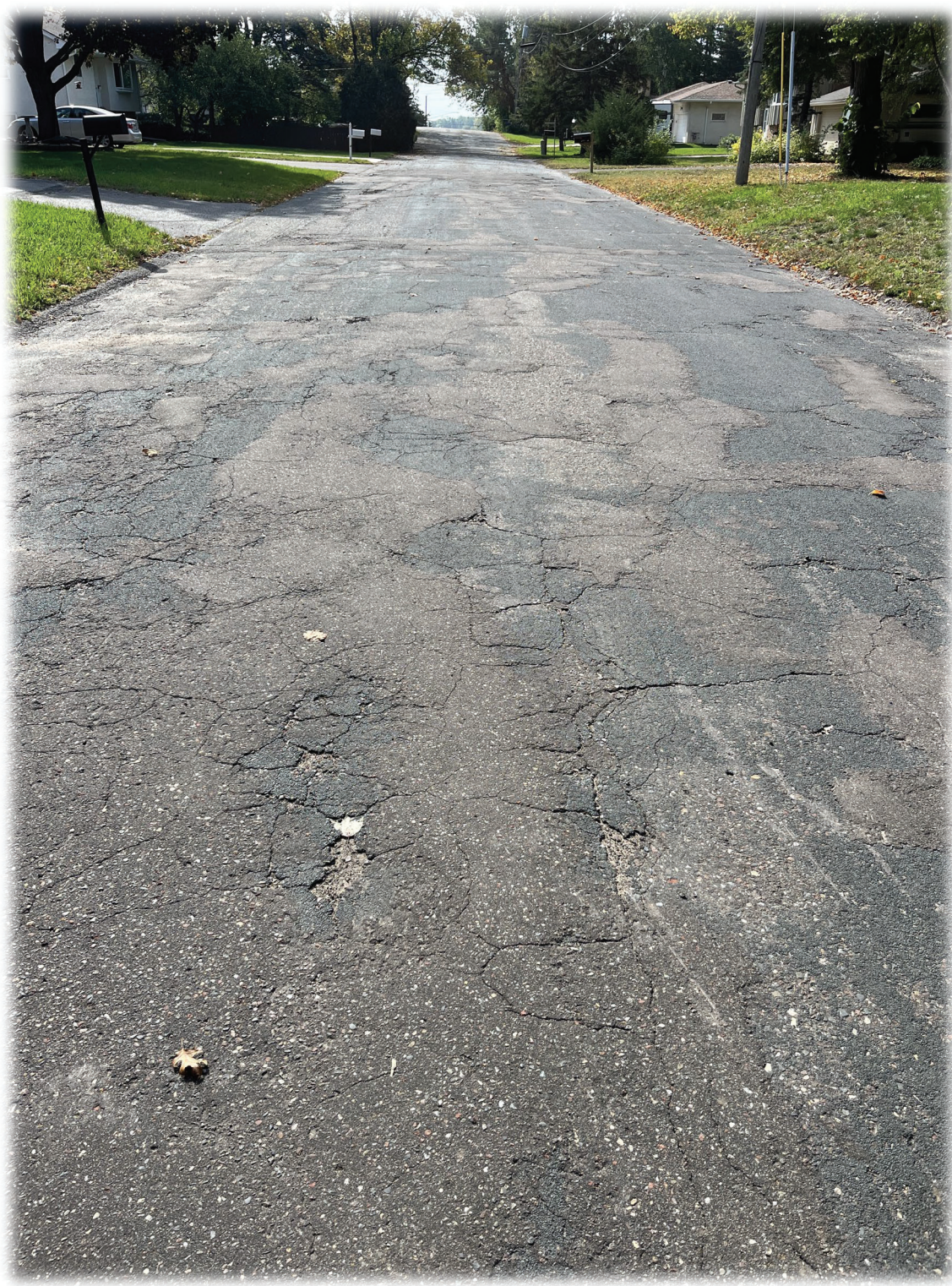
FIGURE 1: Pavement Condition of the East Shore Drive Area Streets
