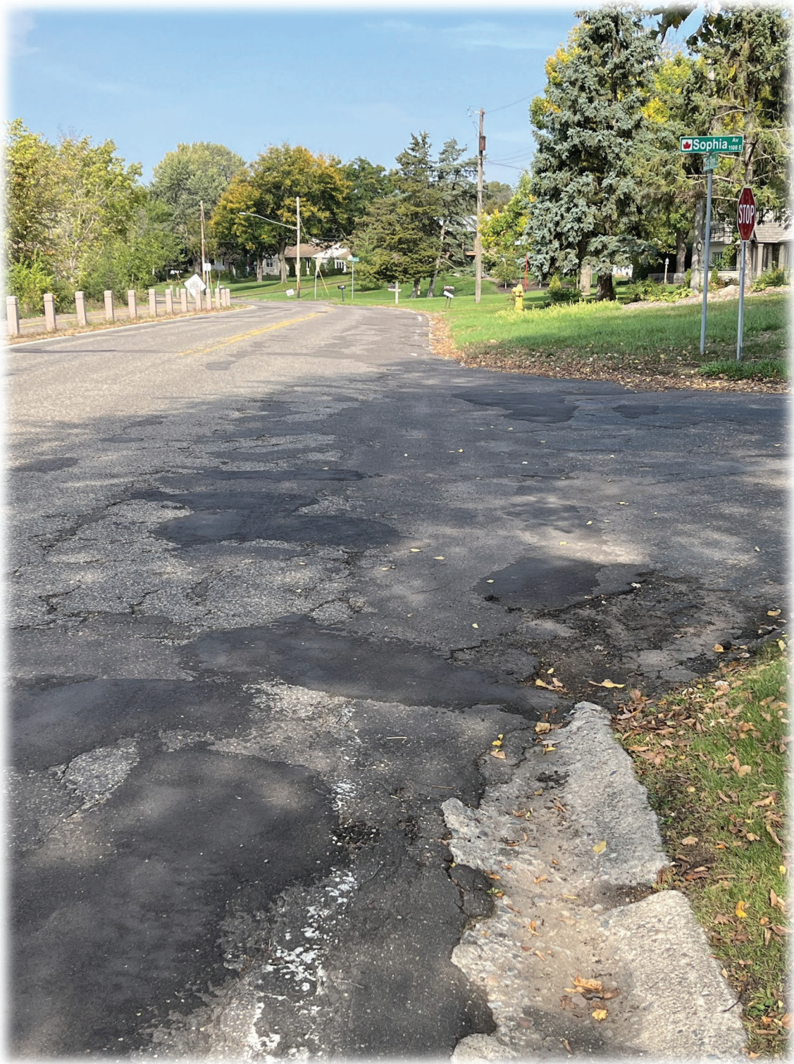
FIGURE 2: Pavement Condition of the East Shore Drive Area Streets
