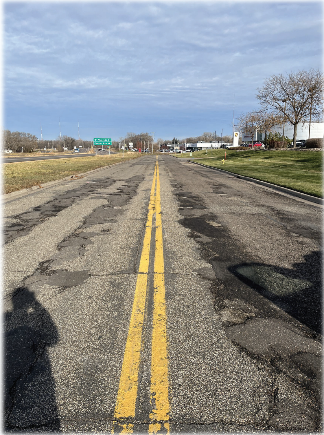
FIGURE 4: Pavement Condition of the Cypress-Maplewood Drive Area Streets
