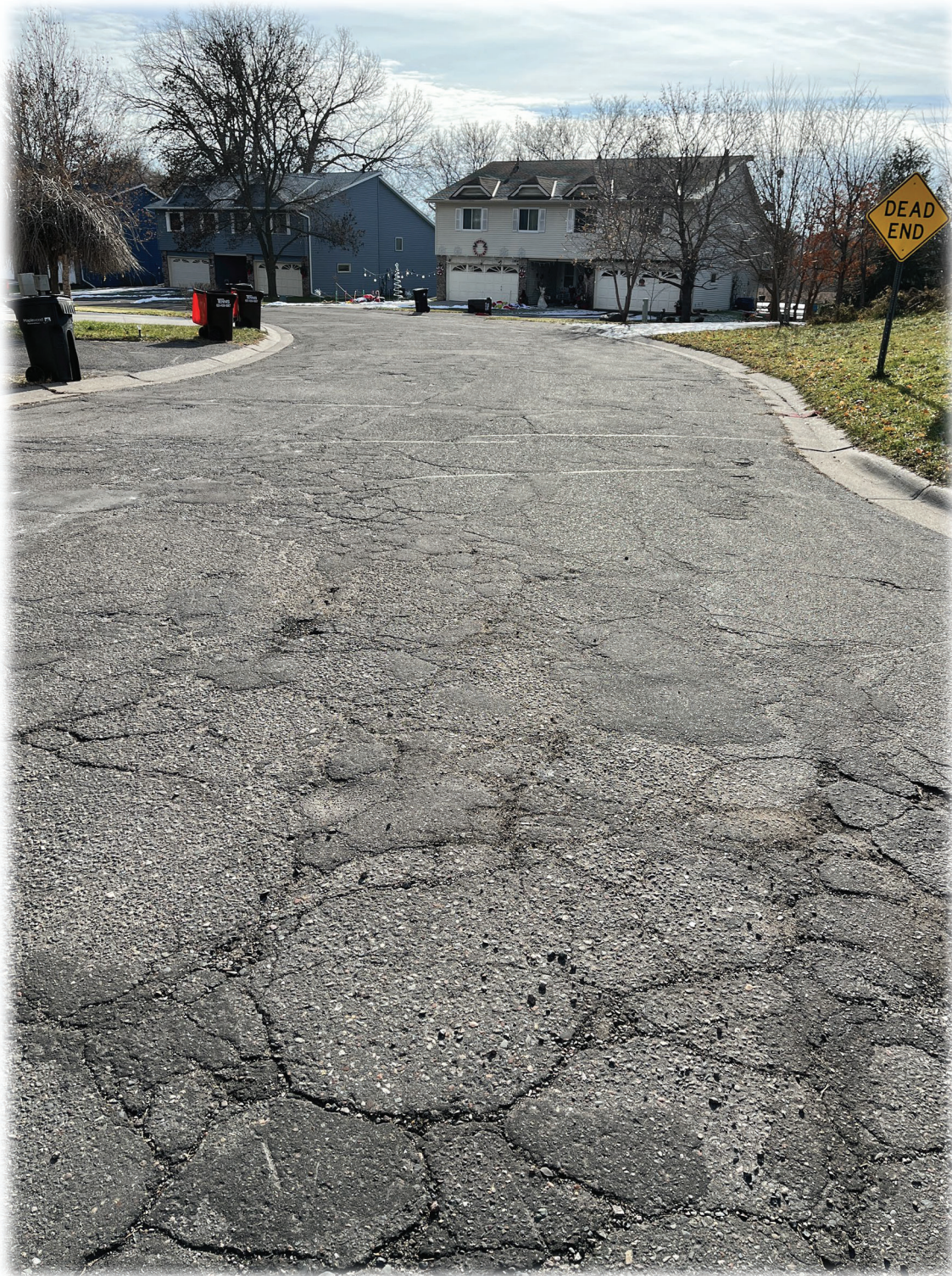
FIGURE 7: Pavement Condition of the Cypress-Maplewood Drive Area Streets
