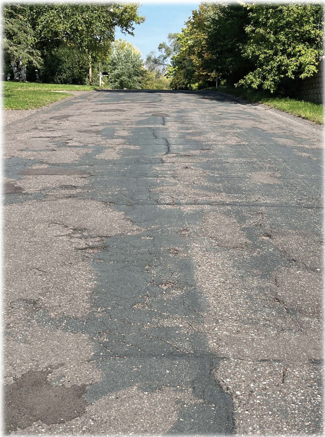
FIGURE 6: Pavement Condition of the East Shore Drive Area Streets
