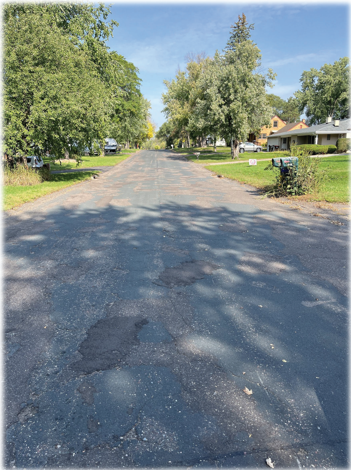
FIGURE 4: Pavement Condition of the East Shore Drive Area Streets
