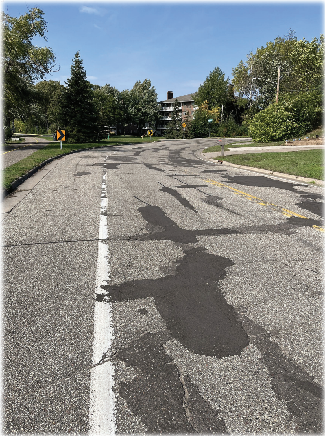
FIGURE 8: Pavement Condition of the East Shore Drive Area Streets
