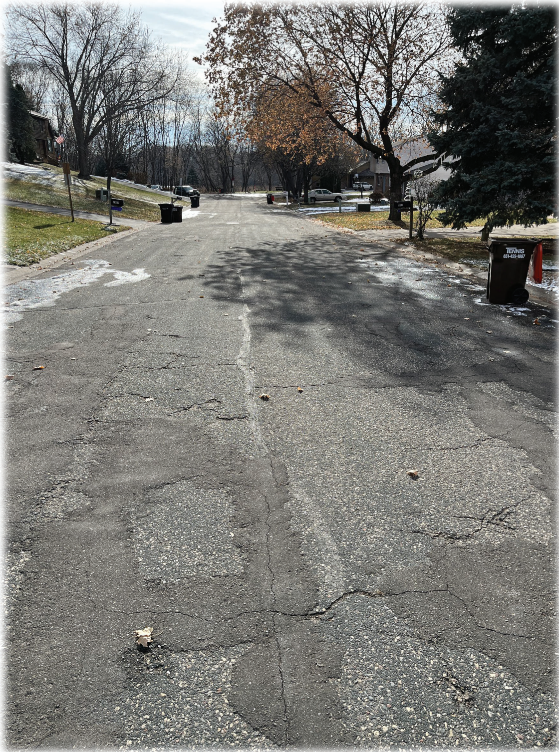
FIGURE 5: Pavement Condition of the Cypress-Maplewood Drive Area Streets
