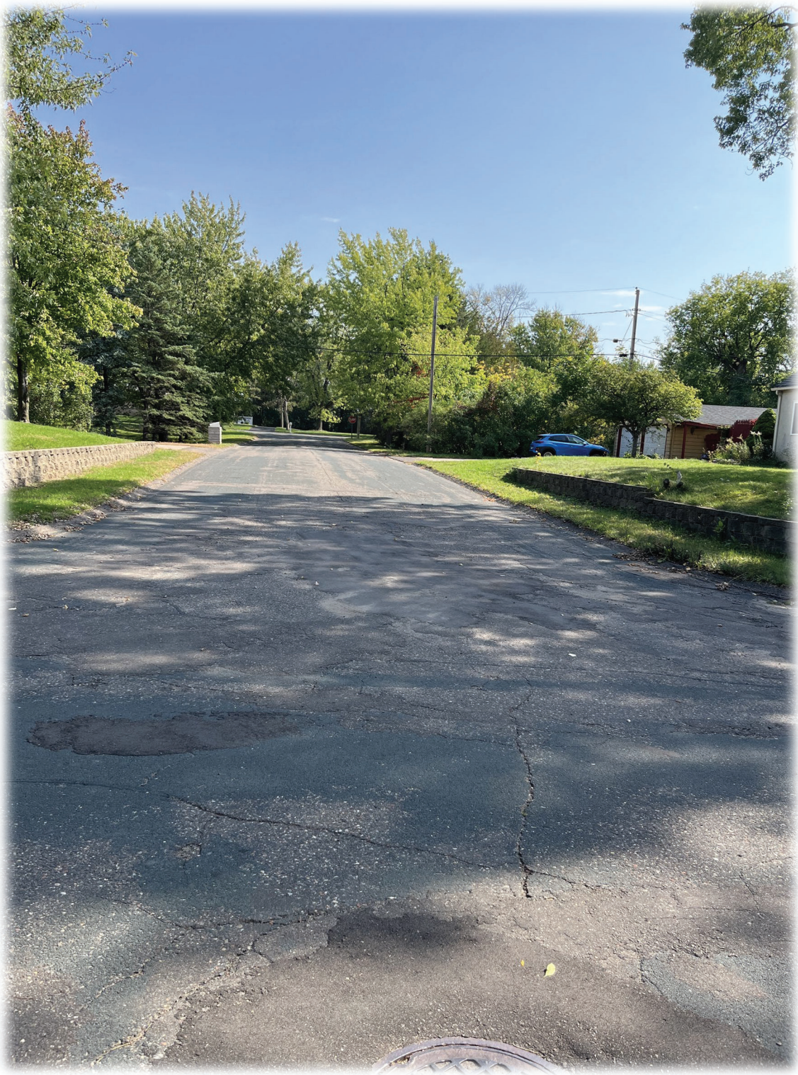
FIGURE 7: Pavement Condition of the East Shore Drive Area Streets
