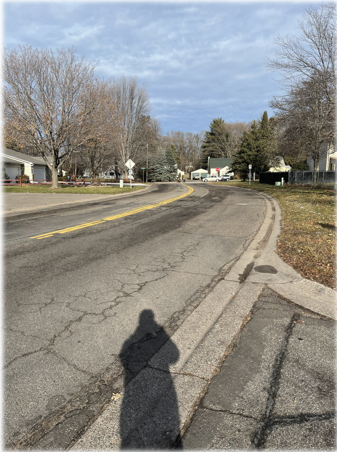
FIGURE 6: Pavement Condition of the Cypress-Maplewood Drive Area Streets
