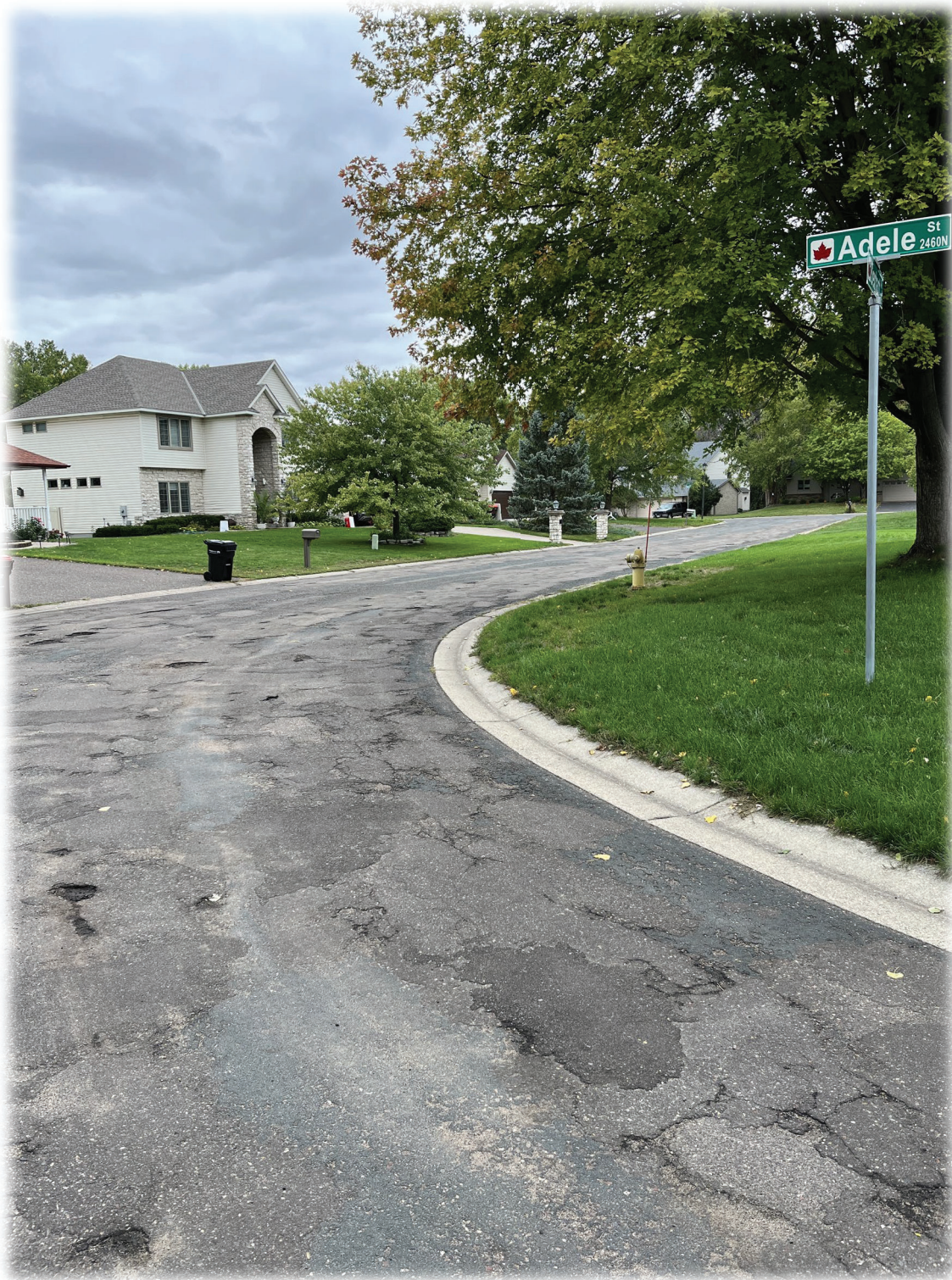
FIGURE 3: Pavement Condition of the Cypress-Maplewood Drive Area Streets
